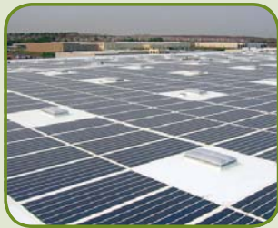
Solar Panels on Distribution Center in Riverside, CA
